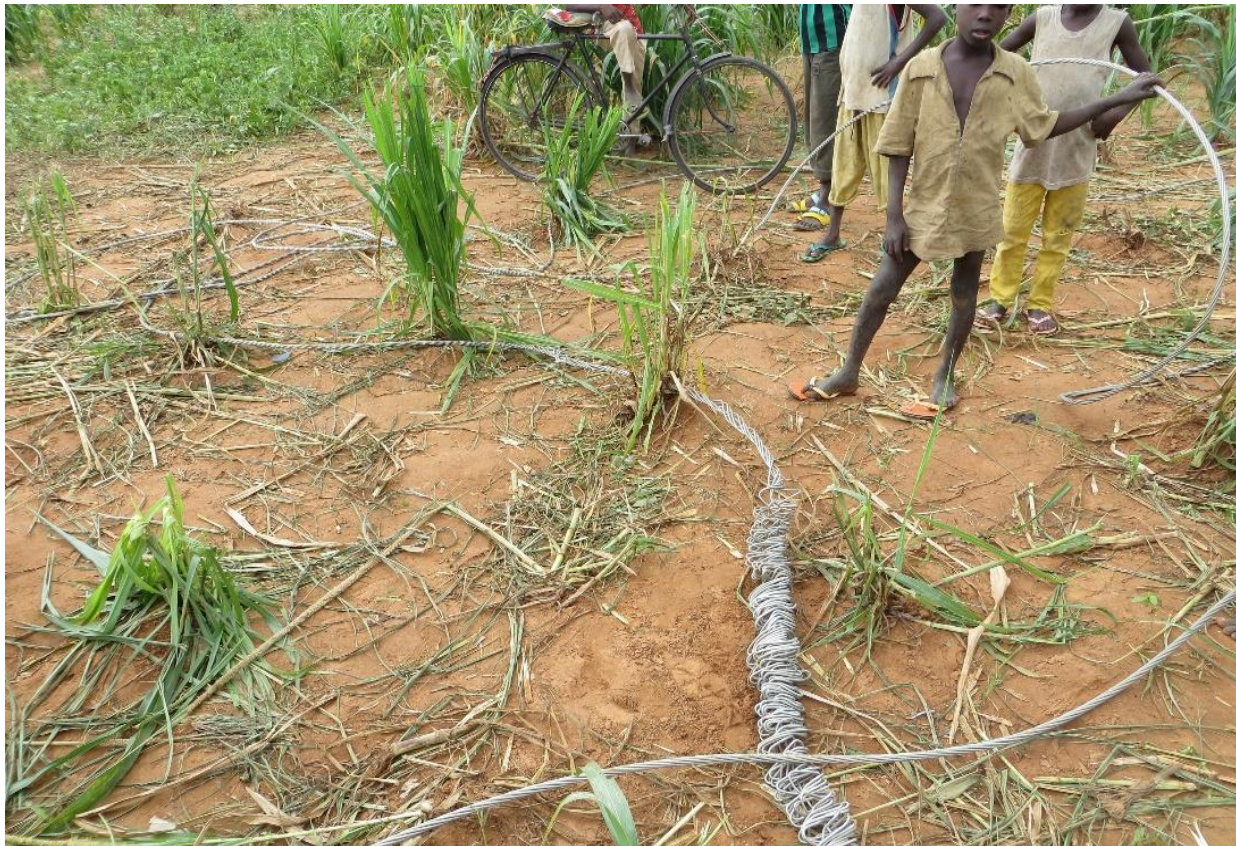
Figure 4: Snapped Electricity Cables
