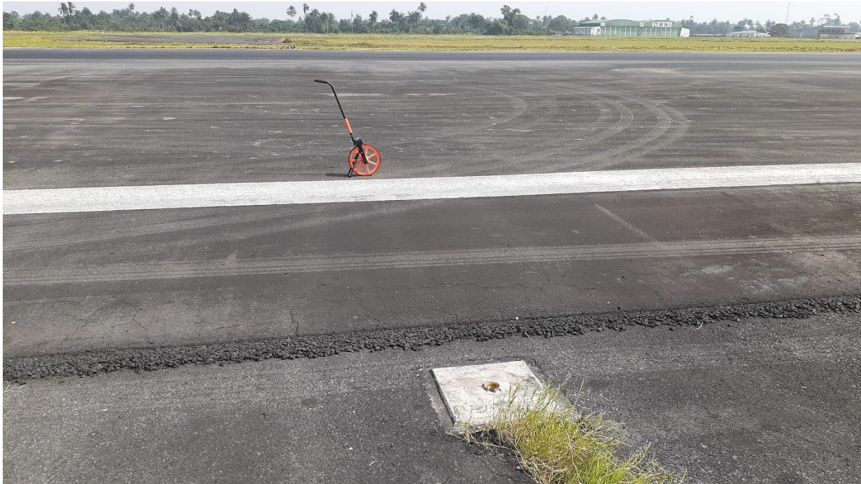
Figure 5: Photo of one of the damaged runway edge lights
