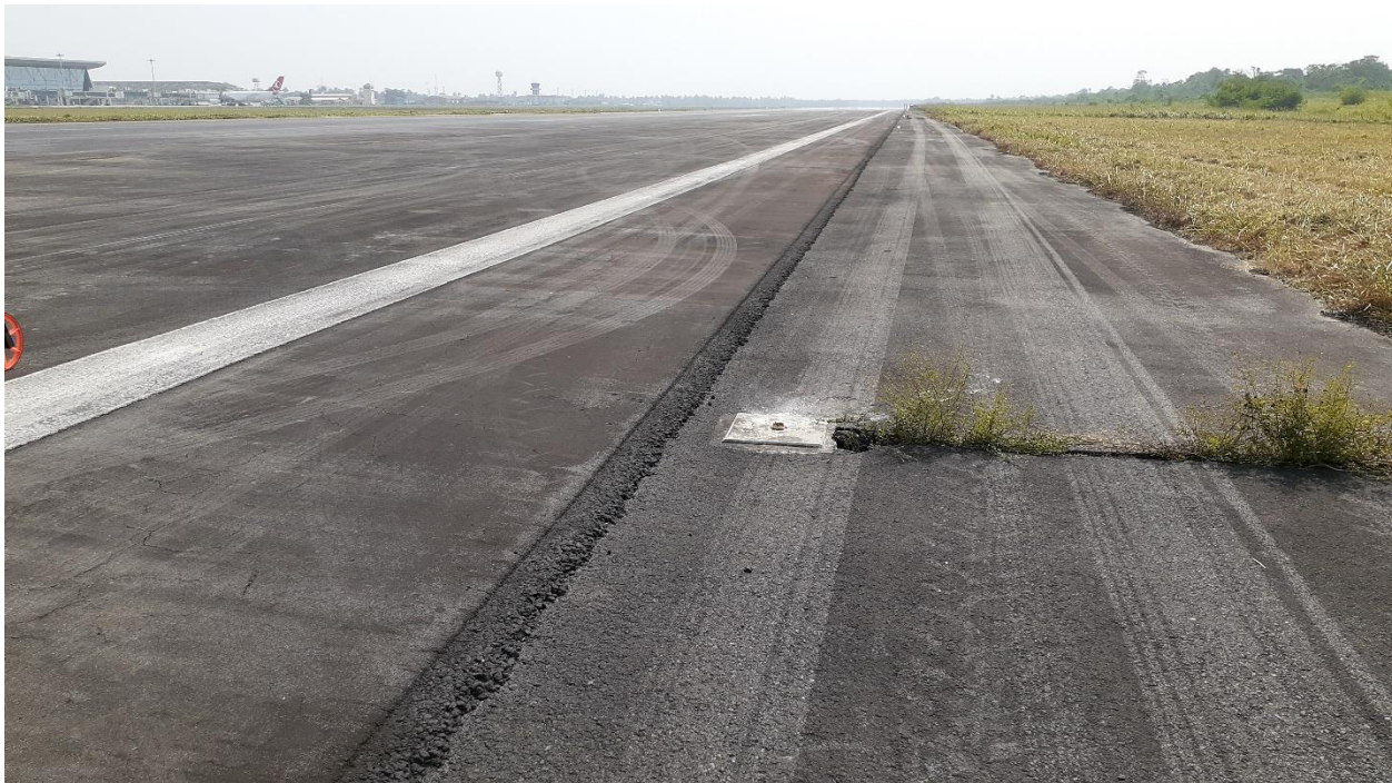
Figure 6: A photo of the tyre marks from the right main wheel tyres on the runway shoulder
