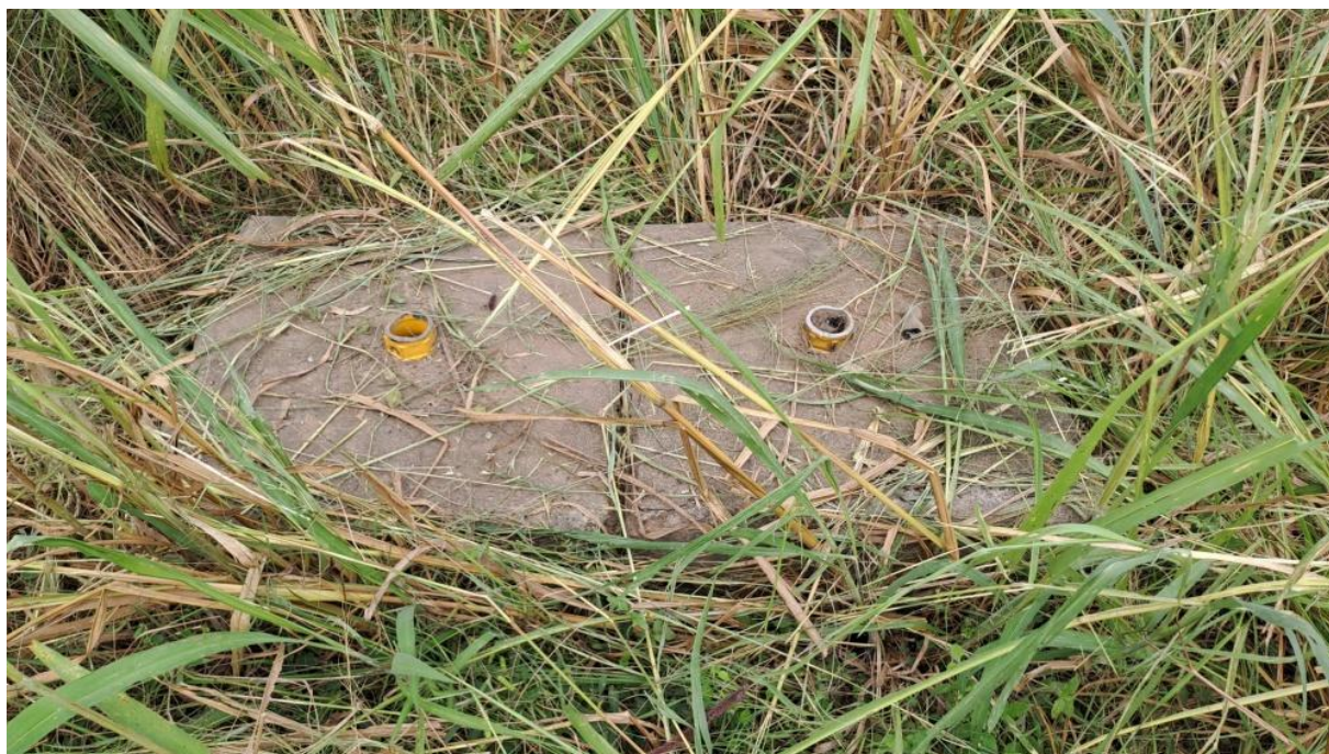
Figure 3: Some of the decapitated runway approach light fittings
