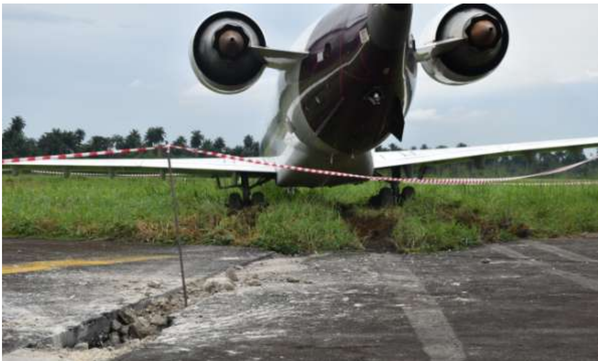
Figure 2: The damaged drainage duct (In the foreground)
