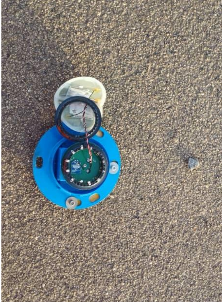
Figure 1: Picture of broken taxiway edge light
