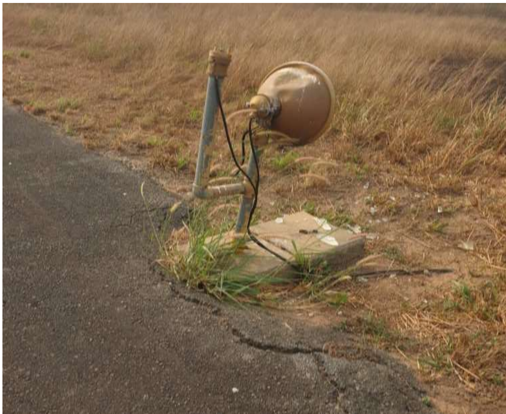
Figure 3: Back view of the broken approach light on runway 22 end
