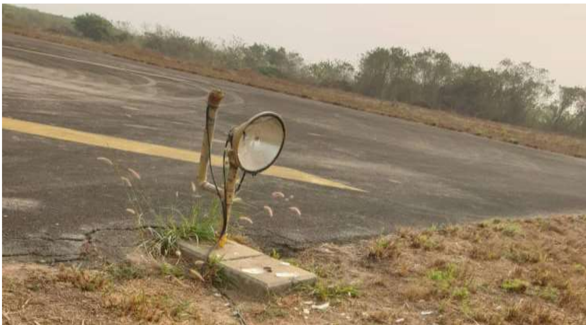
Figure 4: Front view of the broken approach light on runway 22 end
