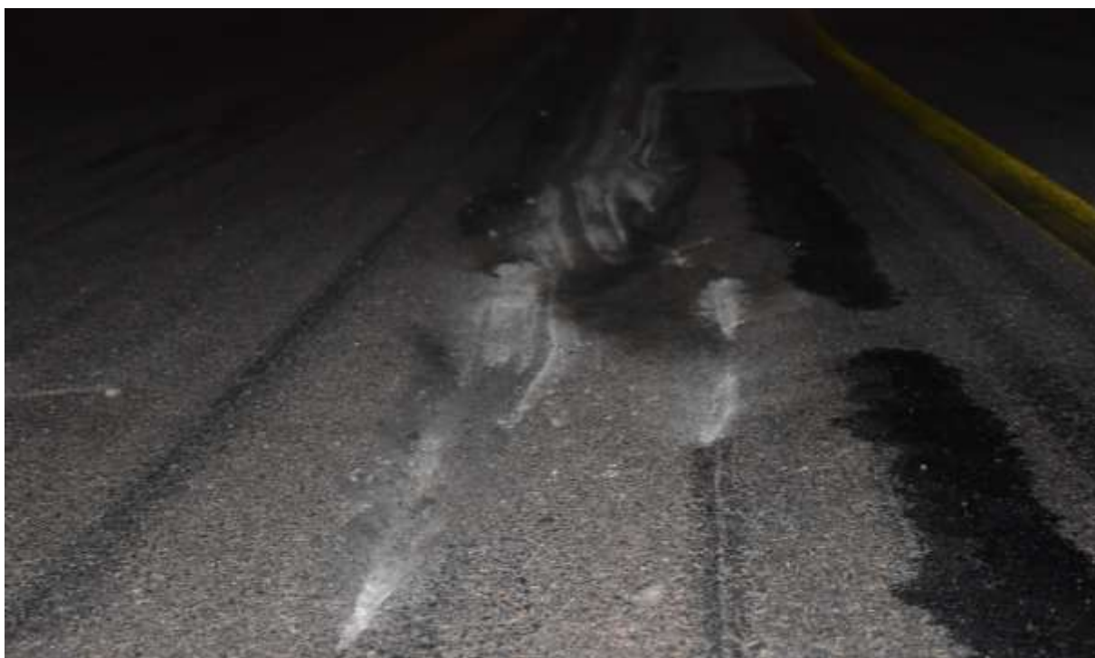
Figure 2: Scratch marks on the runway surface
