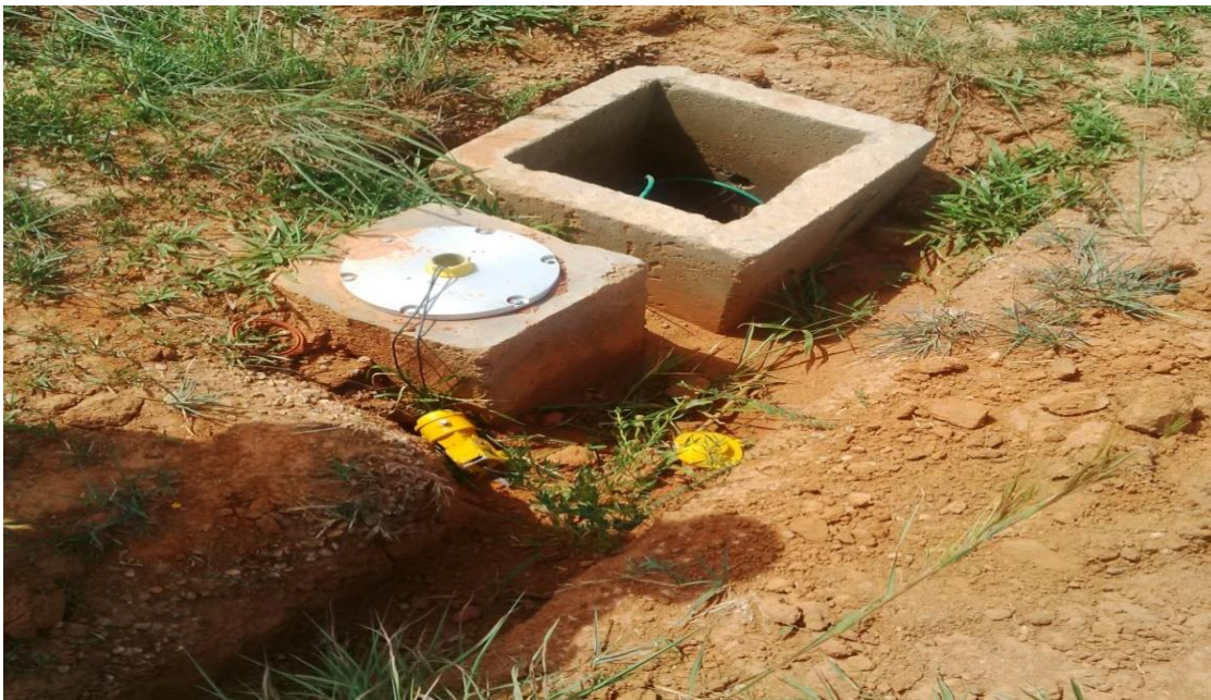
Figure 2: Damaged approach lights
