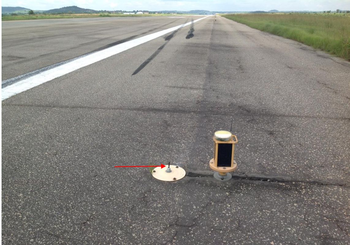
Figure 5: Damaged runway edge light
