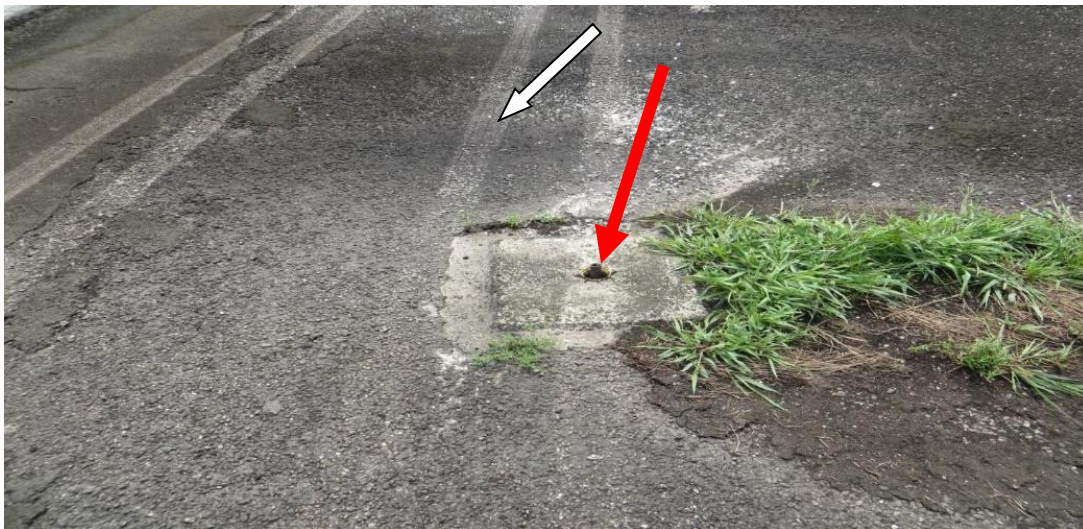
Figure 3: The main wheel tyre marks on the runway right shoulder (white arrow) and a damaged runway edge light (red arrow)
