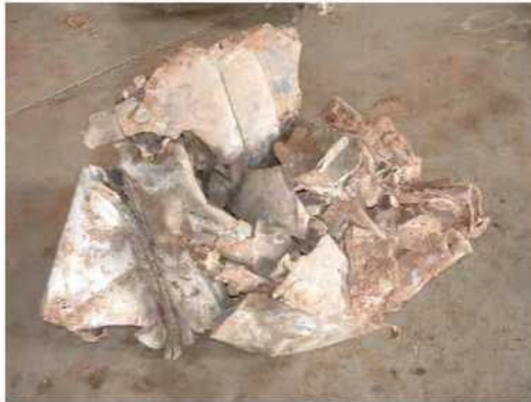
FIG 8 – Fwd Cargo Door Cutout Lower Sill Area
