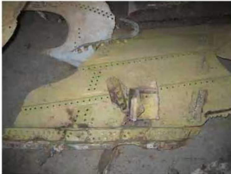
FIG 48C Pieces of LH outboard wing box lower skin at WBL 103 and rear spar. View looking down and forward.
