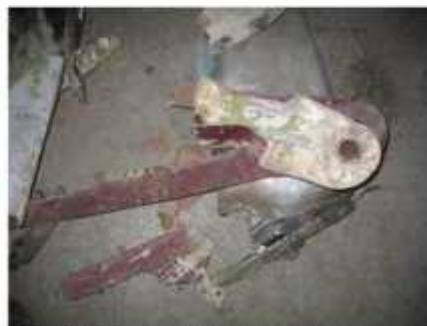
FIG 60B LH main landing gear support beam outbd end – split on bond line.
