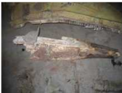
FIG 60C RH main landing gear support beam outbd end. Smoke and/or heat damage on the outbd end.
