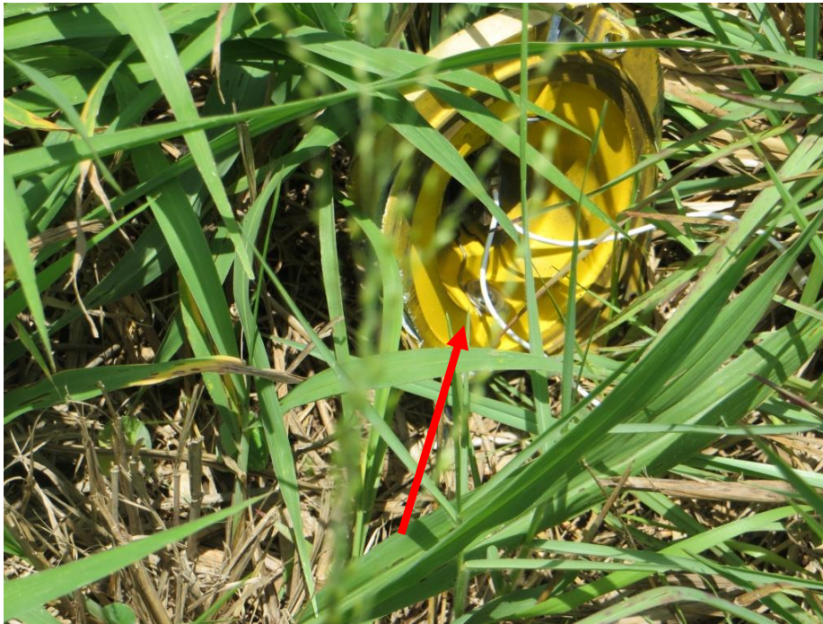
Figure 2: Photo of the broken runway edge light fixture
