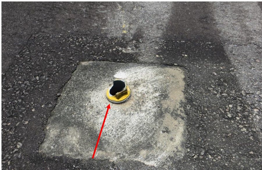
Figure 1: A broken runway edge light fixture base
