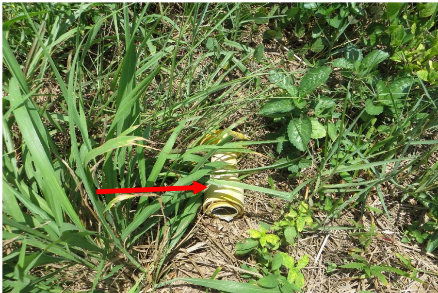
Figure 3: Photo of the broken runway edge light fixture
