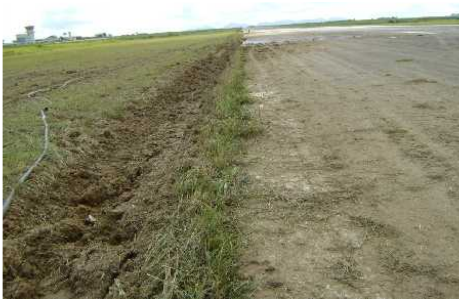
Fig 1.12g Picture showing tyre marks of aircraft veered off the runway 28 and up-rooted armored cable
