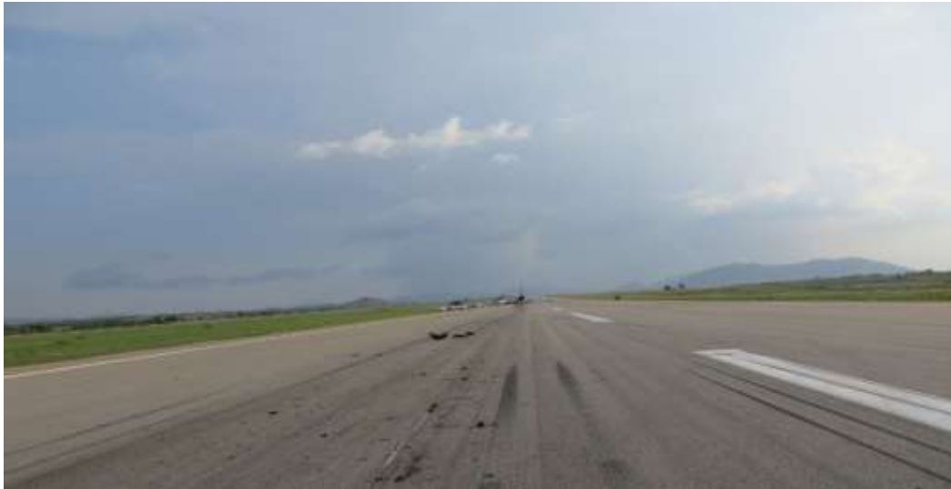
Figure 5: Debris of the No.2 main wheel tyre
