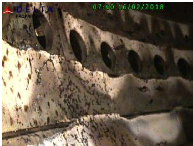
Figure 4: A view of the interior of the combustion chamber showing corrosion
