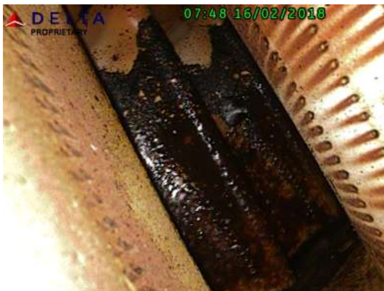
Figure 5: Picture showing corrosion in the turbine section
