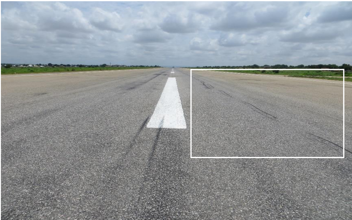
Figure 7: Witness marks indicating Tyre Number 3 failure
