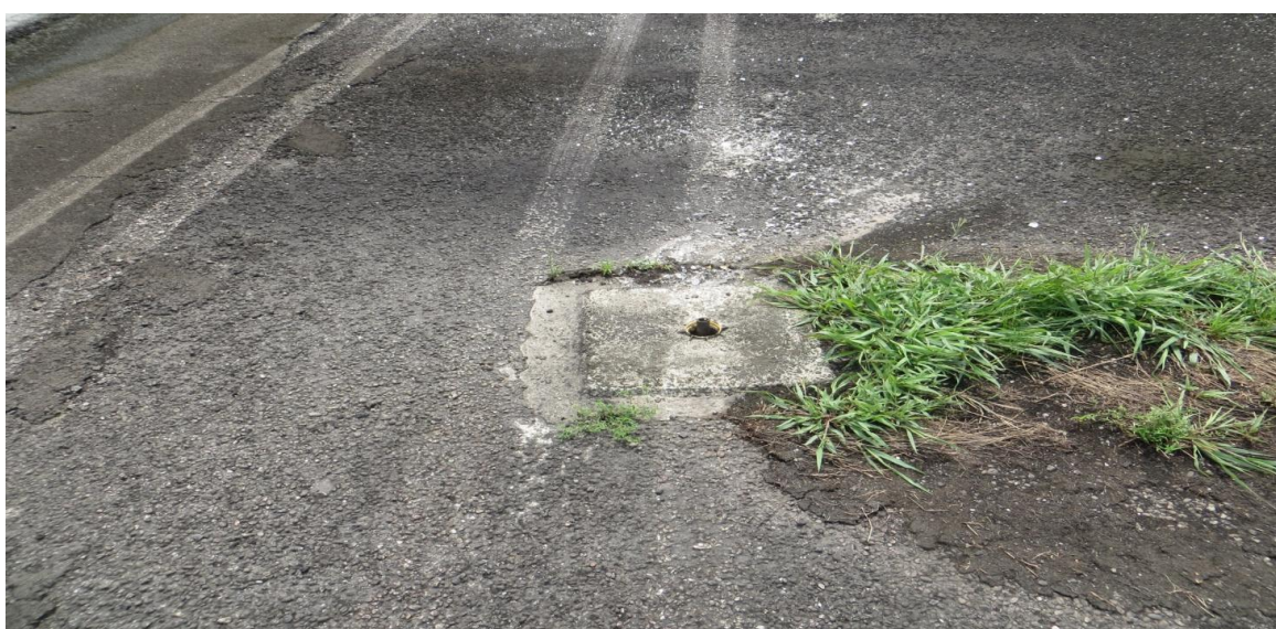
Figure 2: Photo showing the damaged runway edge light
