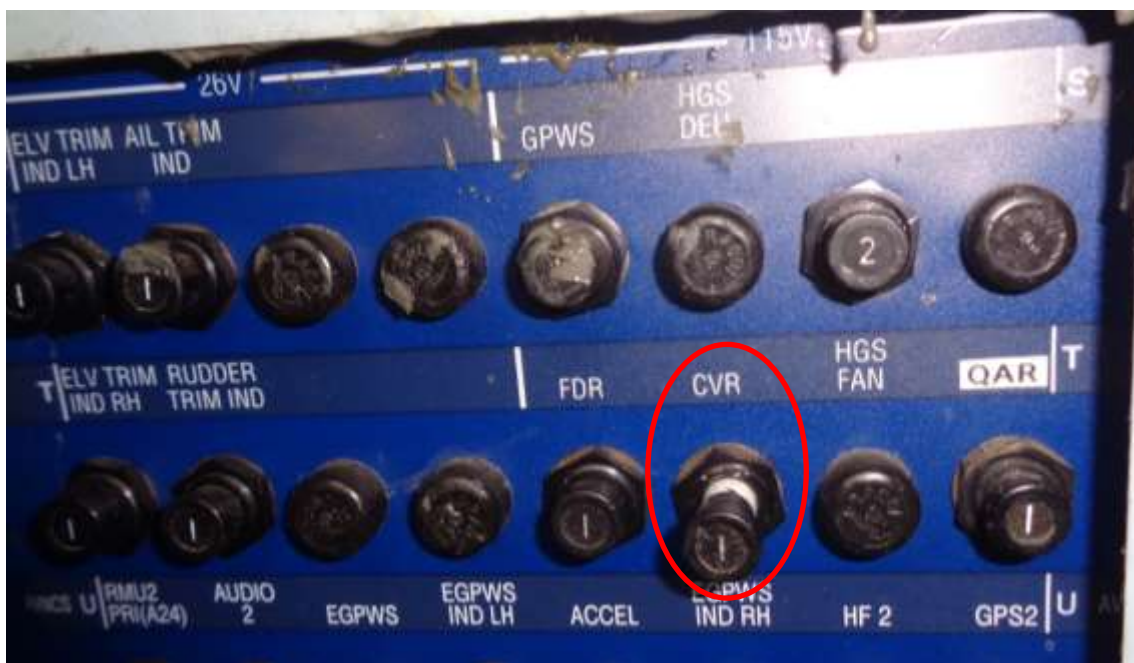
Figure 2: The right side CB panel showing the pulled CVR circuit breaker
