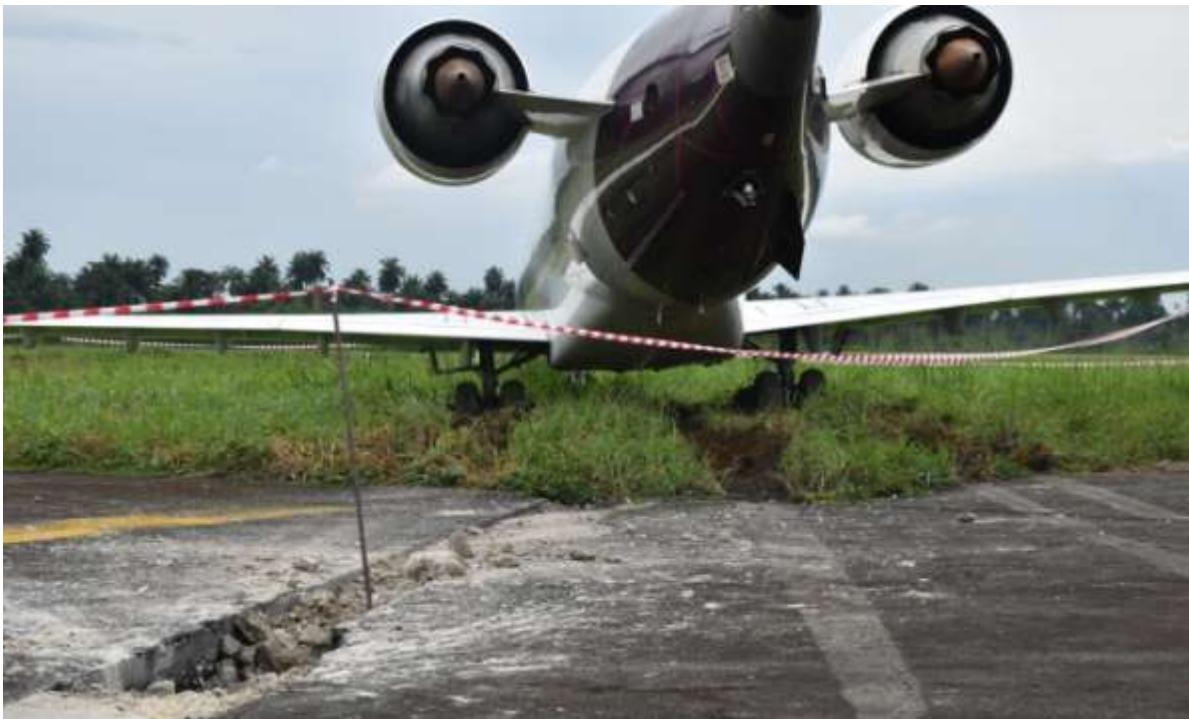
Figure 2: The damaged drainage duct (In the foreground)
