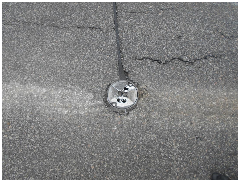
Figure 1: Photo showing witness mark and damage to runway lighting
