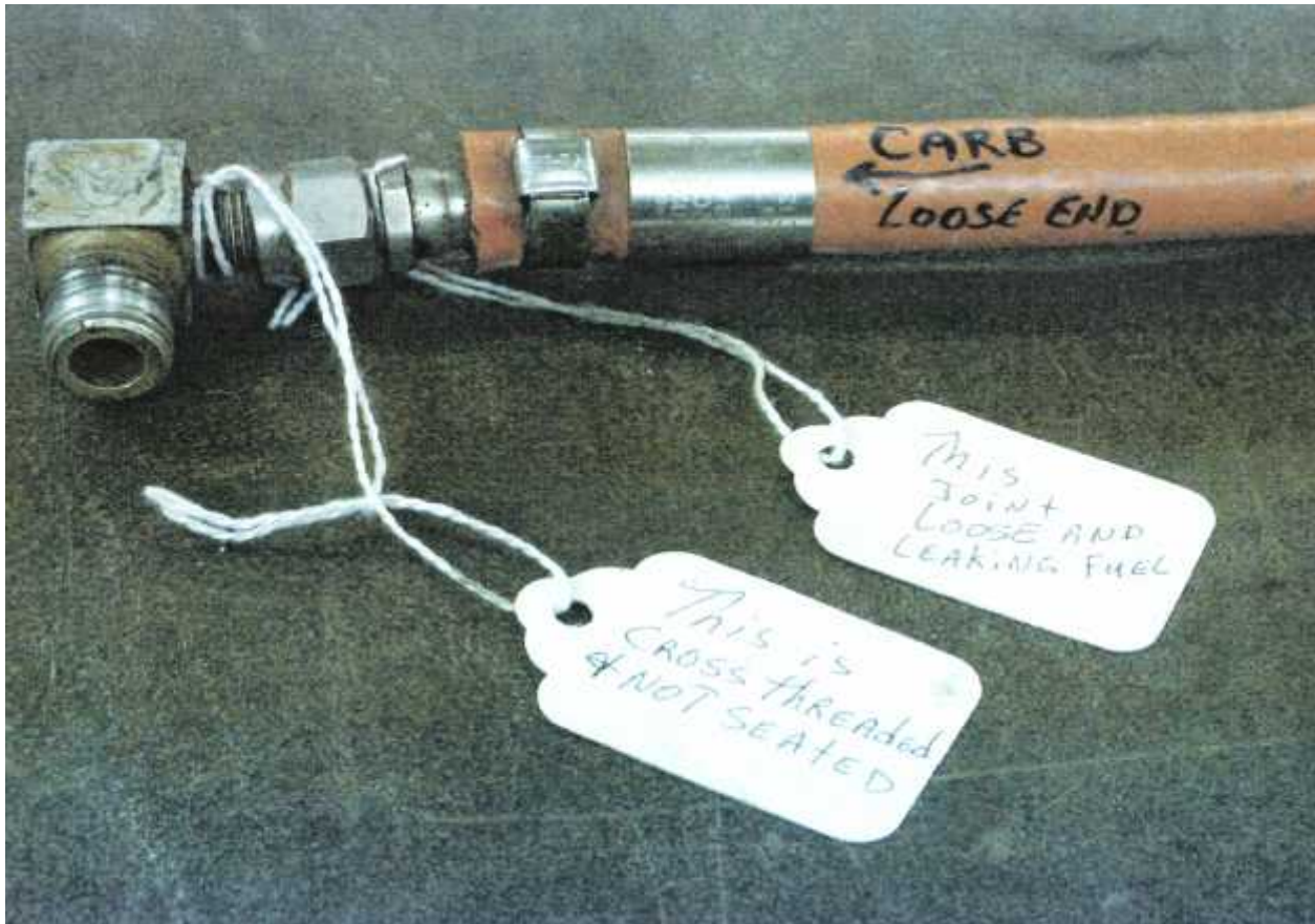
Fig. 1-11 Photograph showing fuel hose and 90° fittings
